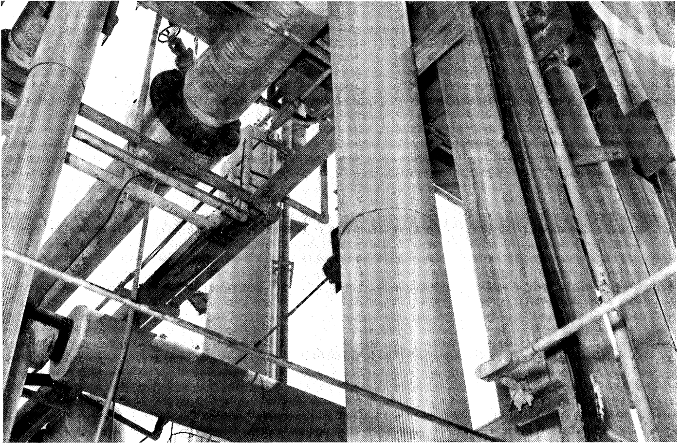
Figure 4. Location of pipeline flange with respect to adjacent piping and instrument tubing.
